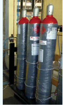
Figure 4.18 : Storage of refrigerant cylinder
